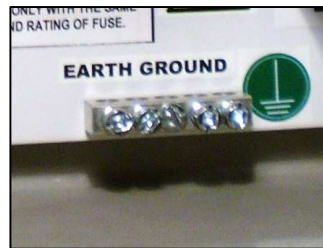
Earth Ground Connection
