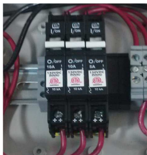
Solar Circuit Breakers
